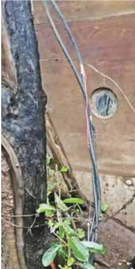
The electricity connection suspected of causing the fatal electrocution.
